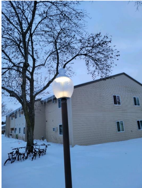
New Parking Lot Lights (LED)
