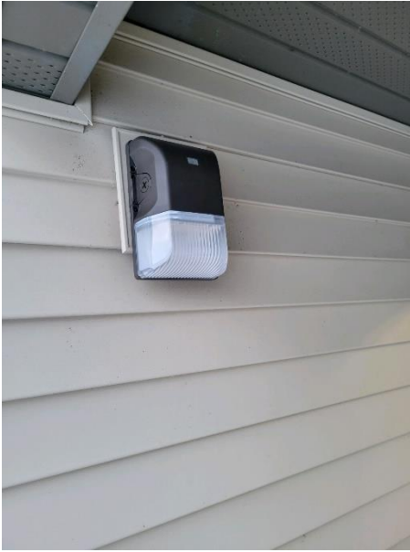
New Exterior Building Lights (LED)
